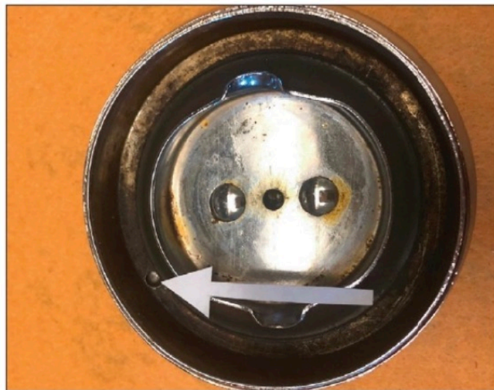
Check for dirty or corroded vent holes.
